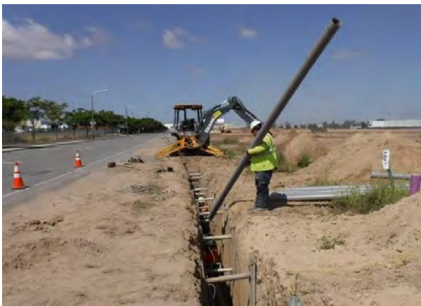
Kitching Substation Feeder Line - Modular 12kV
