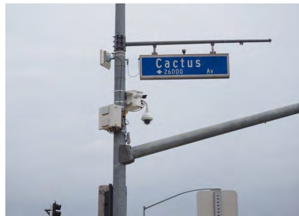
Citywide Camera Surveillance System
