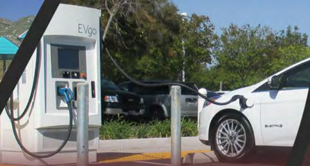
City Hall Electric Vehicle Charging Station
