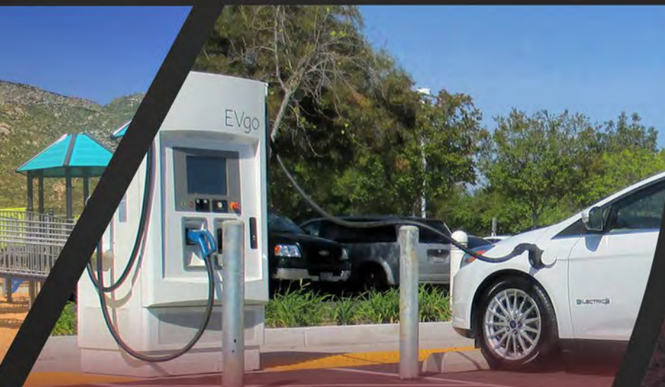
City Hall Electric Vehicle Charging Station
