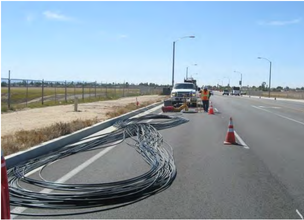
Citywide Fiber Optic Communications Expansion
