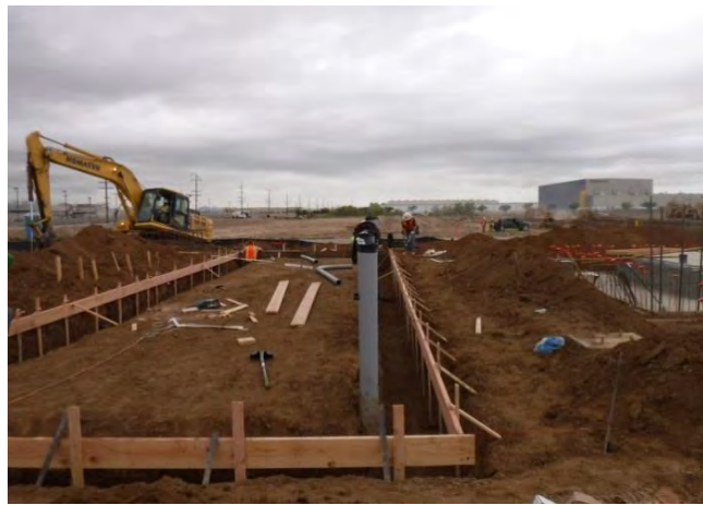
Kitching Substation and SCE Switchyard / Facility Upgrades
