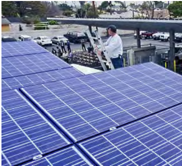
Solar panels on top of the Baldwin Park Unified School District office.
