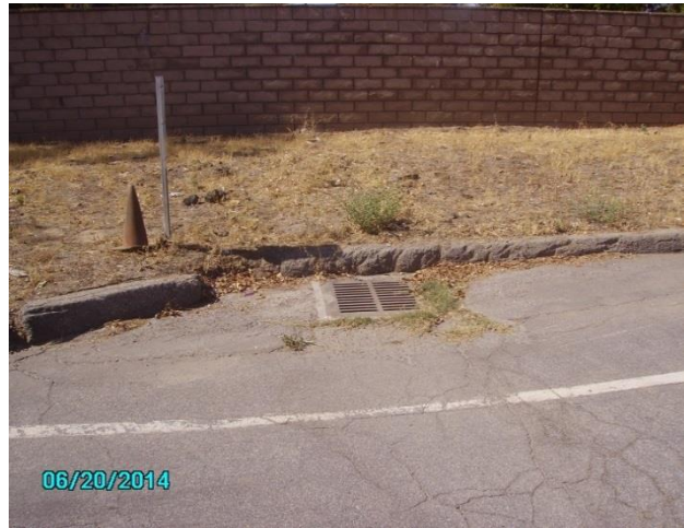
Photo 4: French drain on south side of Kalmia Avenue, approximately midway between Pettit Street and Dow Street.
