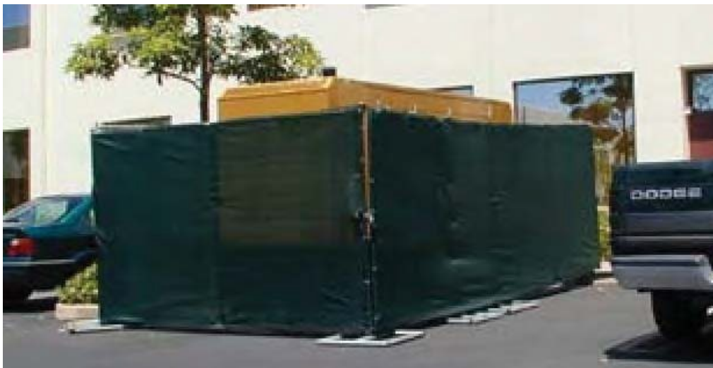
Figure 5-26 Example of Inappropriate Ground Mounted Equipment Screening
